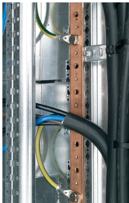
Main terminal in cable sleeve consisting of a 32 x 5 mm copper bar
